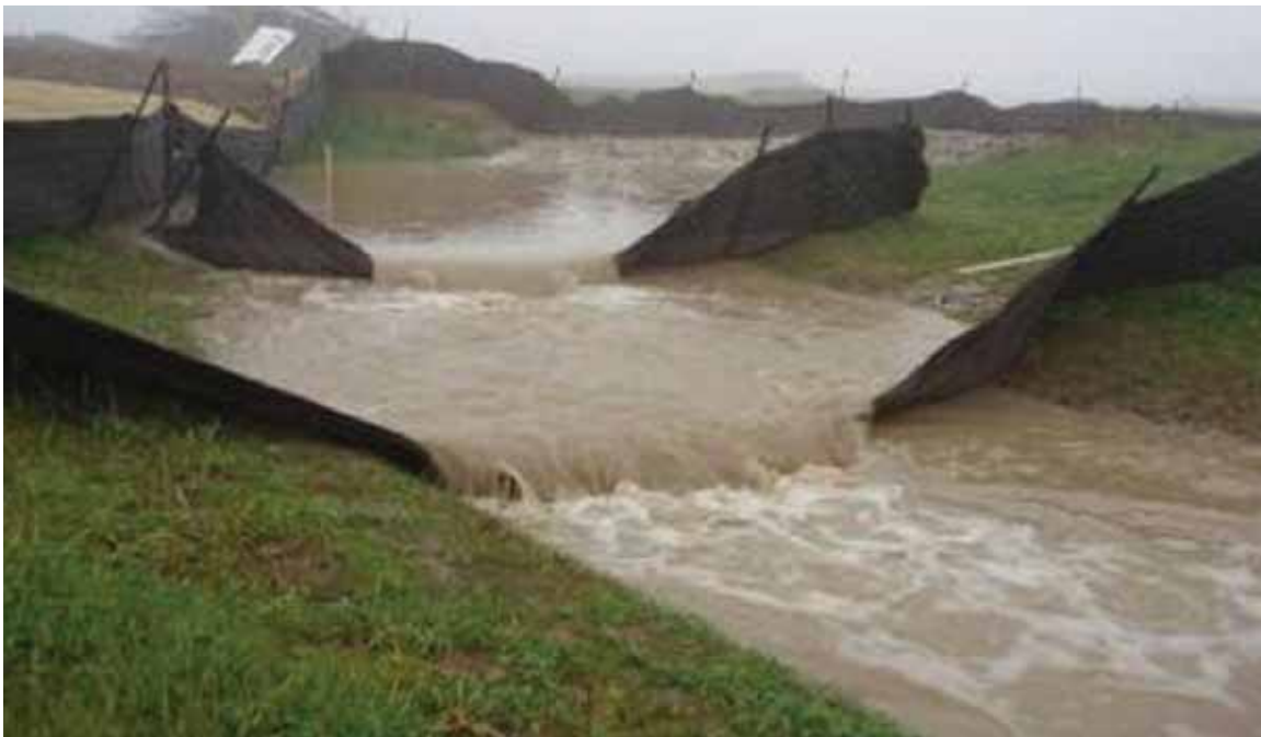
Figure 17: Erosion from a construction site
