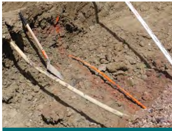
Figure 4.1.2: Utilities are major barrier to construction. The pipes pictured above were not listed in the background information and caused construction delays as excavation had to work around them. (Source: CVC)
