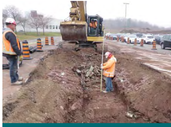
Figure 9.2.2: In this photograph, the contractor is verifying the depth of excavation while under supervision. (Source: CVC)
