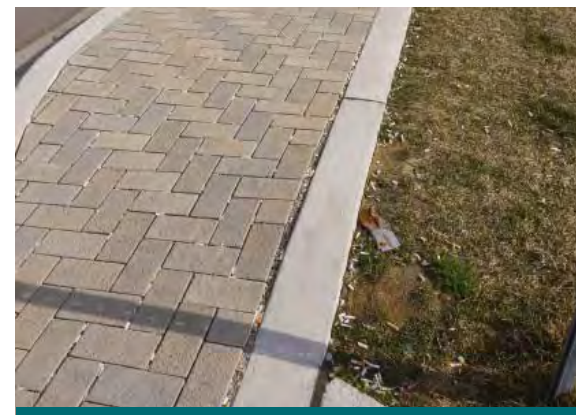
Figure 4.9.1: Further consideration of user behaviour may have resulted in a different LID solution for this location. This section of sidewalk is a preferred smoking location for the adjacent business and the cigarette butt waste stuck between the permeable pavers will be an ongoing maintenance problem. (Source: CVC)
