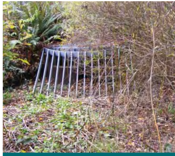
Figure 6.4.13: A grated ditch inlet catch basin can be used at the downstream extent of a bioswale. (Source: Aquafor Beech)
