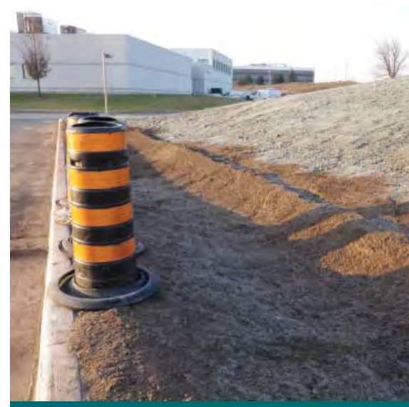
Figure 9.3.2: Approved bioretention soil media is installed at the IMAX Project site. (Source: Aquafor Beech)
