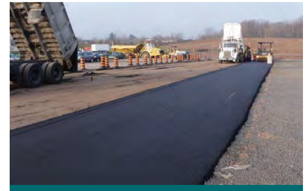
Figure 9.6.4: A temporary asphalt road used for construction access is one way to reduce onsite erosion caused by constant traffic from heavy vehicles and equipment. (Source: Aquafor Beech)
