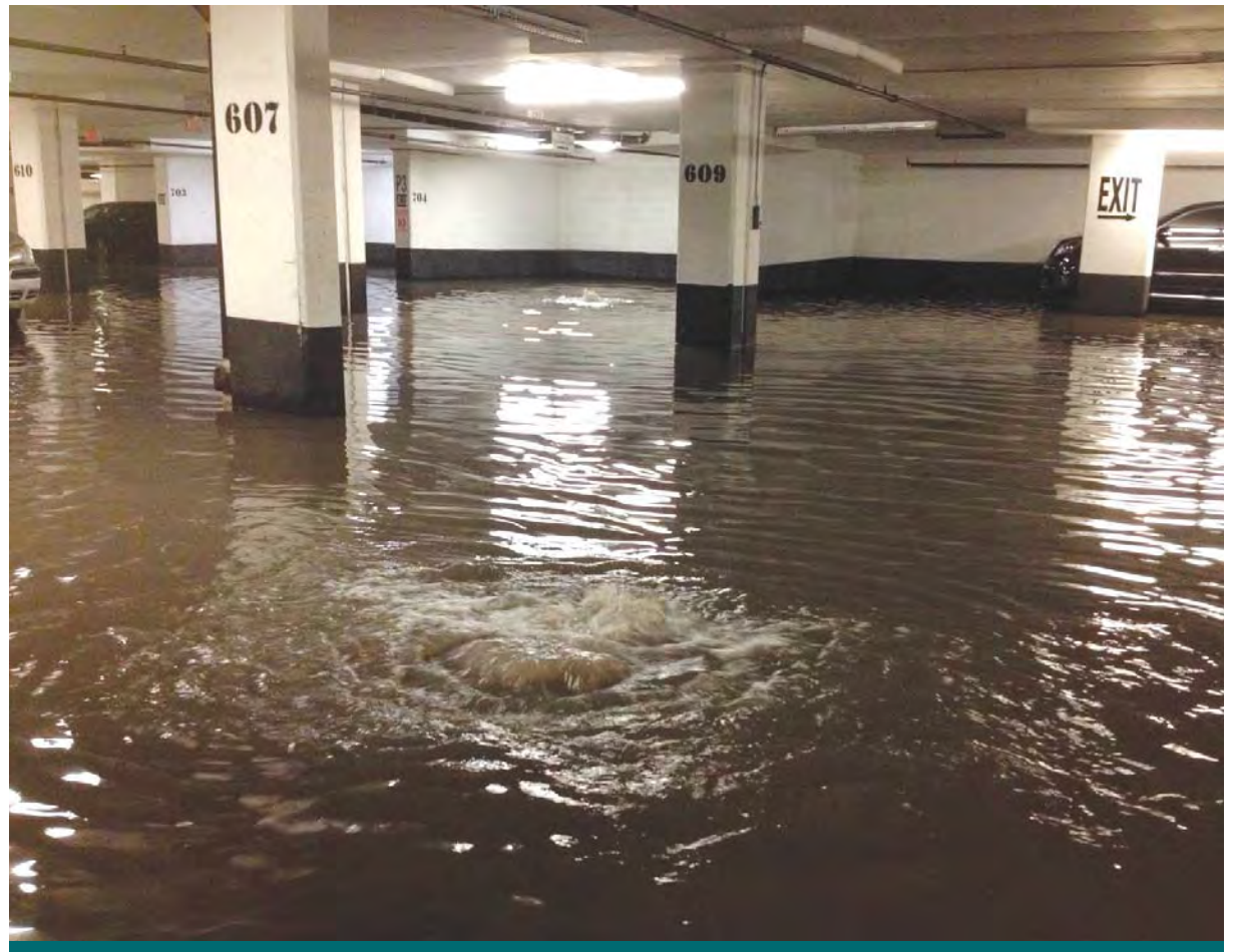
Figure 11.0.1: Reducing risk is another indicator of project success. An apartment building in Mississauga was evacuated due to structural deficiencies as a result of the July 8, 2013 flood. Improved site drainage can prevent costly infrastructure failures and may avoid insurance premium increases. (Source: CVC)
