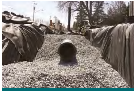
Figure 2.6.1: A perforated pipe is installed in a granular trench to encourage infiltration. (Source: Aquafor Beech)
