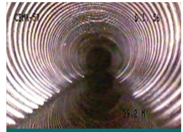
Figure 10.2.4: Video inspection (pipe scoping) is a rapid means of identifying issues with buried pipe. Look for indications of pipe collapse, blockages, or sediment buildup. This photograph from an Ottawa perforated pipe shows it to be in excellent condition even after more than 20 years of performance. (Source: City of Ottawa)
