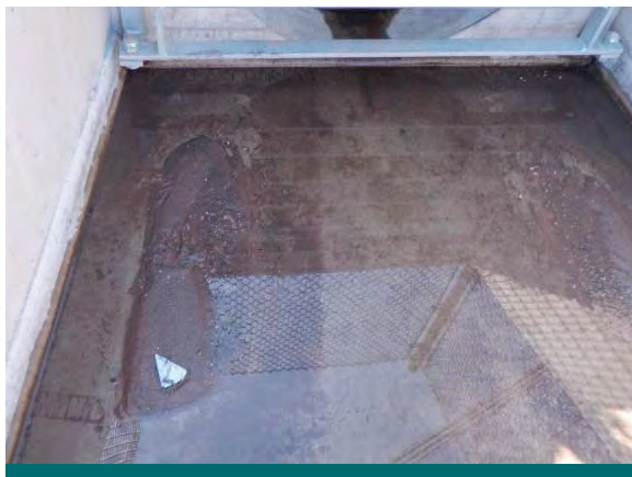
Figure 10.2.6: Along with measuring sediment depth in a proprietary stormwater treatment device, check the outlet structure (if accessible). If the device is functioning as intended this sedimentation should not be occurring, unlike this device. (Source: Aquafor Beech)
