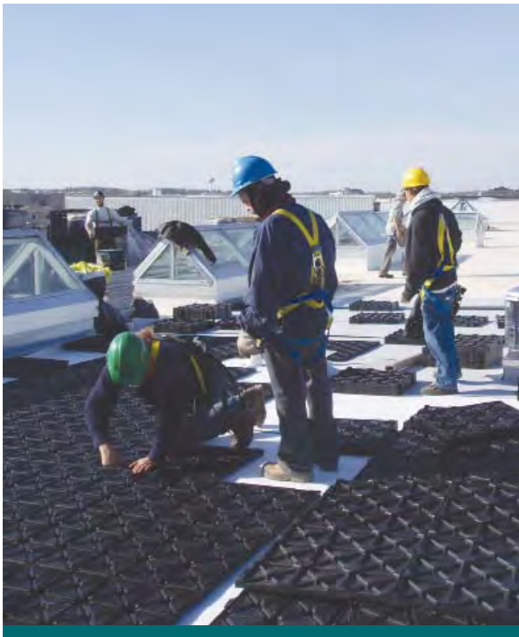
Figure 9.5.1: Mechanical and structural components may interfere with installation on flat roofs. Here contractors work around ventilation components and skylights. (Source: CVC)
