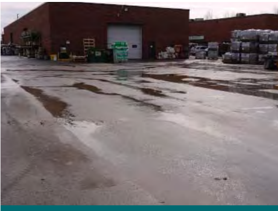
Figure 4.1.4: Improper surface grading can reduce a site's drainage capabilities. At this site, most rainfall causes significant ponding and interferes with day-to-day operations. (Source: CVC)
