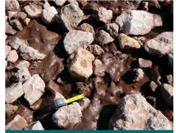
Figure 10.2.3: Closely inspect any pre-treatment areas for excessive sediment accumulation from exposed soil during construction. In this photo a riprap spillway between the forebay and bioretention facility has been subject to clay deposition from upstream construction practices. (Source: Aquafor Beech)
