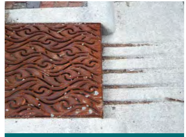
Figure 6.4.11: Inlets with grooves etched into the gutter and concrete apron help slow and direct runoff into LID practices. (Source: Aquafor Beech)
