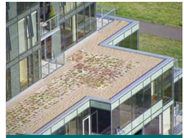
Figure 4.3.2: A tiered rooftop presents unique retrofit opportunities on mid and high rise sites. Tiers can be thought of as catchment areas and can be used as pilot projects before implementing the entire roof area of the building. Here a green roof allows condo owners to have a landscaped front yard, even on the 15th floor. (Source: Aquafor Beech)
