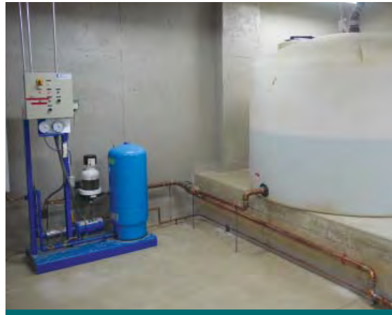
Figure 2.7.1: Rainwater can be stored in a variety of different locations, either outdoors or indoors. For instance, CVC's rainwater storage tank is located in the basement of its head office. (Source: CVC)
