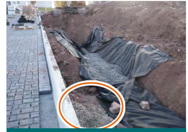
Figure 9.2.3 The granular base of the permeable pavers extends into an adjacent trench constructed for a perforated pipe system installed during the IMAX Project. In the design, the two features were to be hydraulically separated by a clay plug. (Source: Aquafor Beech)
