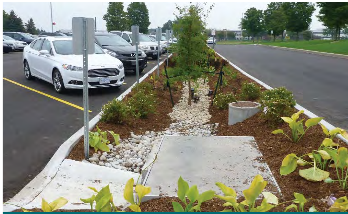
Figure 6.4.22: A Jellyfish® filter pre-treats stormwater within the bioretention area at the IMAX Project site. (Source: Aquafor Beech)
