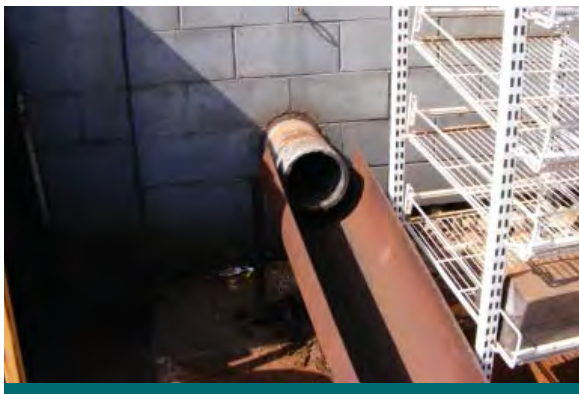
Figure 6.2.2: Here roof drainage is discharged onto the ground surface surrounding a building. This information can be found on mechanical plans. (Source: Aquafor Beech)
