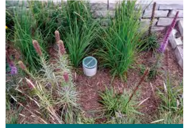
Figure 6.4.14: A plastic flat top overflow is cost-effective but susceptible to damage. (Source: Aquafor Beech)
