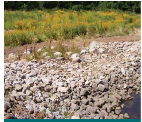
Figure 6.4.21: A stone diaphragm was used at a bioretention area in the Town of Oakville. (Source: Aquafor Beech)
