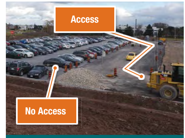
Figure 9.6.3: Consider site function during construction when planning a temporary asphalt road or any other erosion and sedimentation control. (Source: Aquafor Beech)
